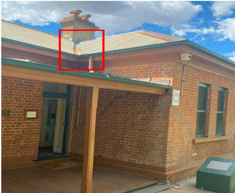
Figure 3 - Due to the eastern section of the building falling away to the east, the valley in the roof has opened and water ingress may be present during rain.
