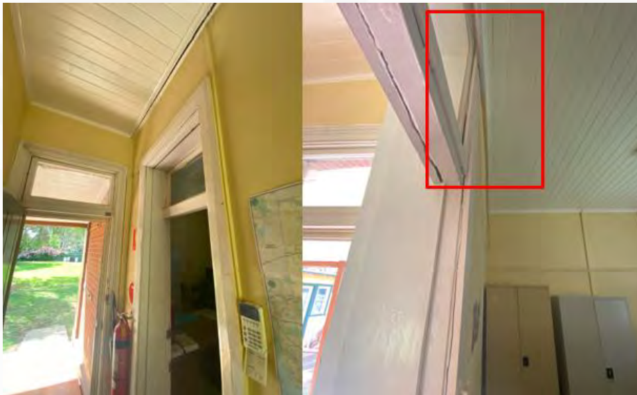
Figure 2 - The western wall of the office room is leaning to the east and is partly being held up by a tension rod on the east of the wall.
