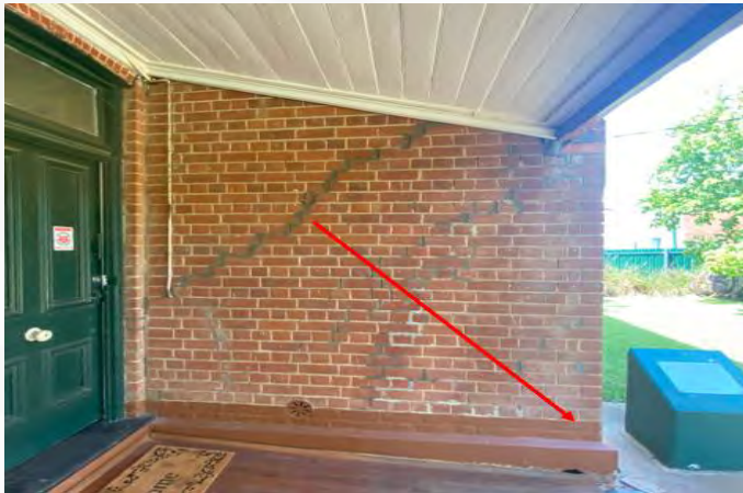
Figure 1 - Repairs at the southern entrance indicate settlement of the footing at the south over time (right in photo)
