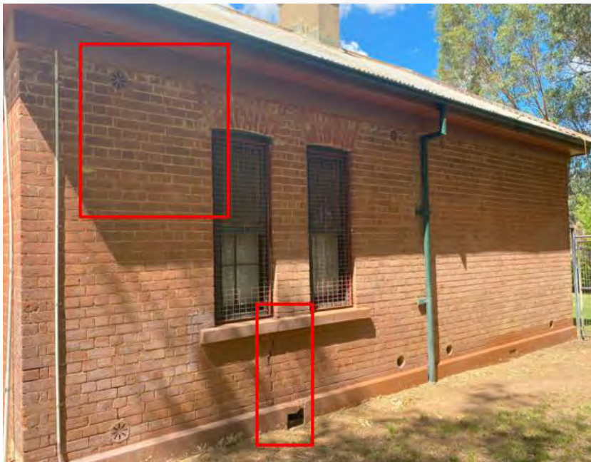
Figure 8 – Cracking throughout the building due to soil movement
