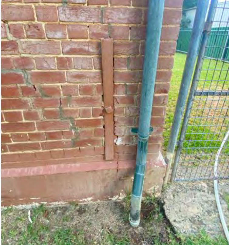
Figure 9 – Tension bracing system is pulling through masonry. The down pipe is not connected to the drainage system.
