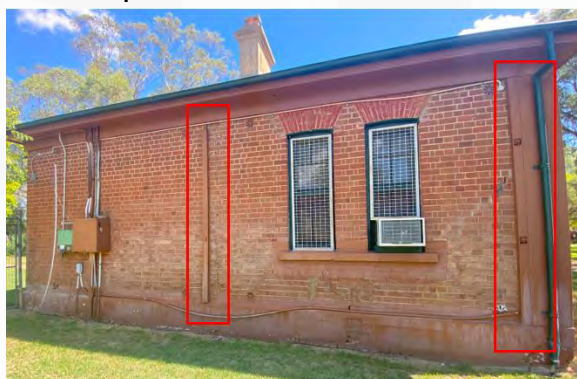
Figure 4 – Eastern wall is leaning east and bulging in the centre. Existing bracing system marked on photo.
