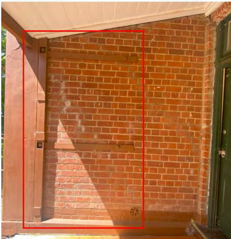
Figure 6 – Significant tension bracing system has been installed at an unknown date to keep the building stable
