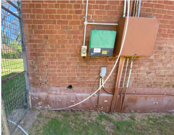
Figure 5 – Southeastern area of the building observed to be the lowest point around the building. Poor drainage and water lying next to footings will contribute significantly to movement of building.
