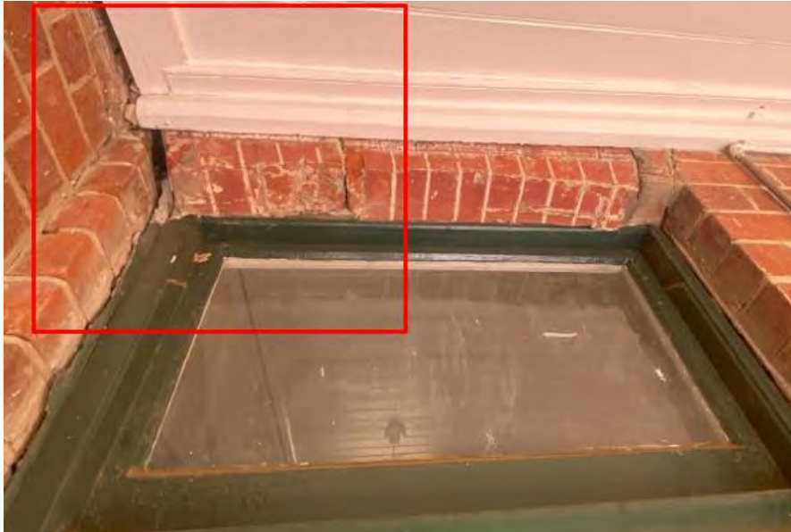
Figure 7 – Eastern section of the building has moved to the east at least 20-30 mm and the door lintel has become unstable
